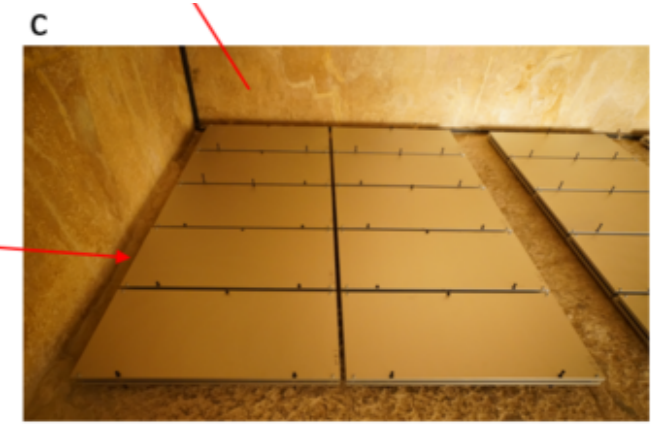
Detectors installed in the Queen's Chamber
