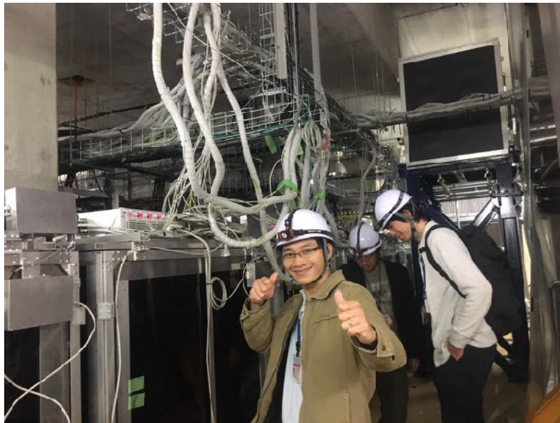
Inside near detector building of T2K experiment, March - June 2019
