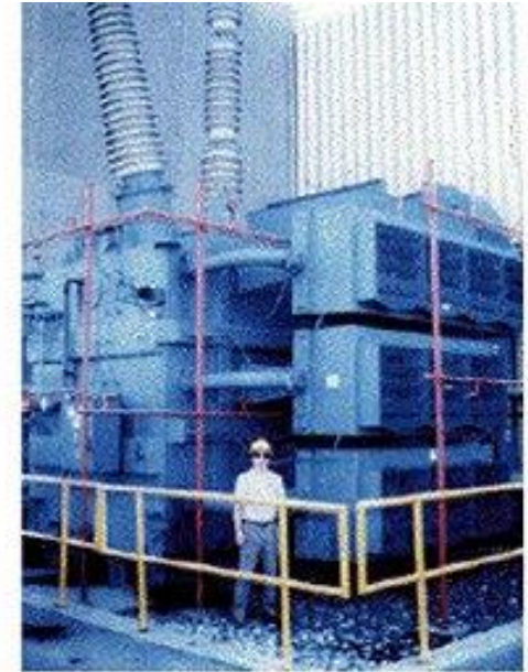
PJM Public Service Step Up Transformer
